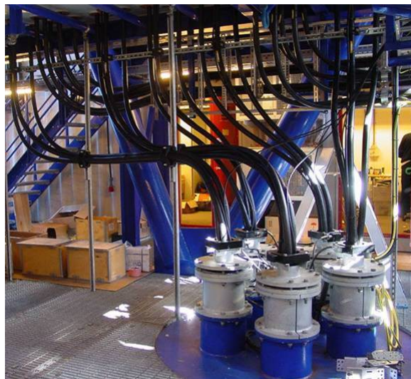
Fig. 7. Inter array 33 kV cables and 150 kV export cable
