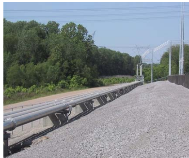
GIL looking north. GIL runs along the road at ground level.
