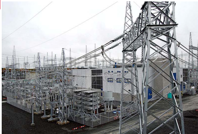
DC filters and DC bus
