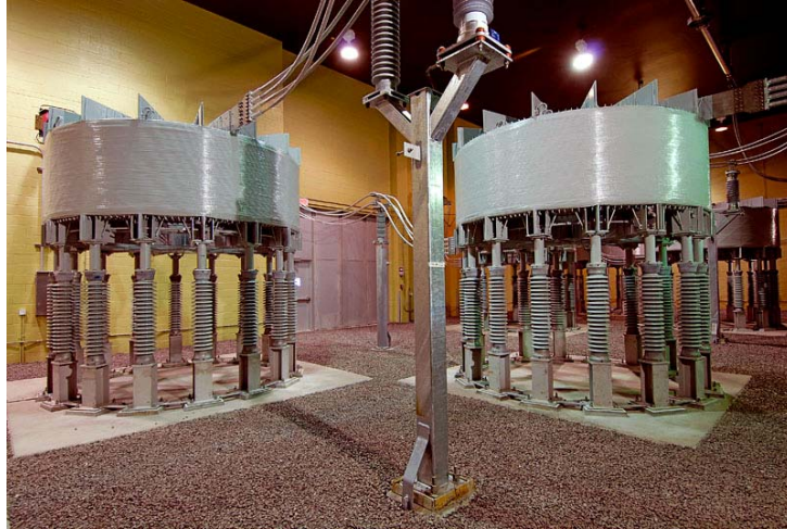
AC coupling reactors
