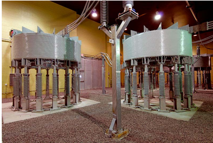
AC coupling reactors
