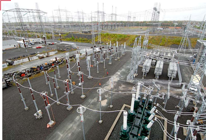
HV connections and transformer
