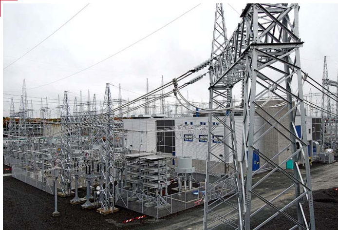
DC filters and DC bus
