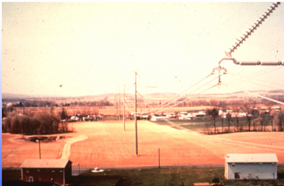
500 kV Horizontal Vee Assembly.
