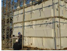
3-D Acoustic for locating source of Partial Discharge
