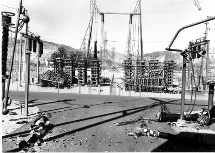
View of the do filters from just outside the building. Note the fallen dividers, capacitor racks, do transformer, and busbars.
