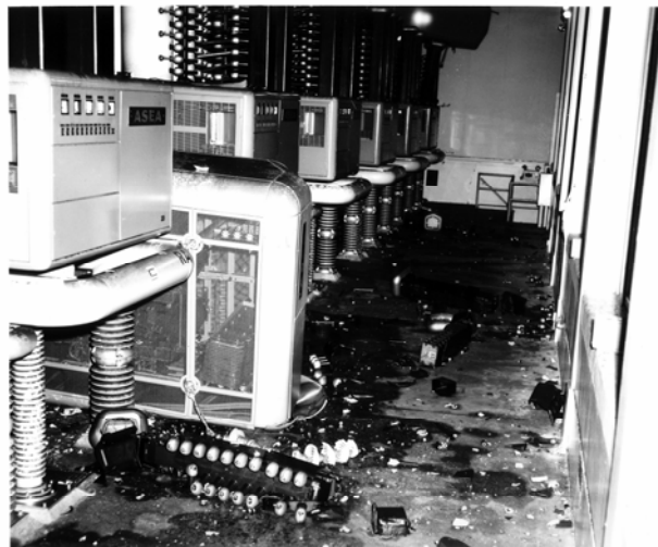
Front view of group 2 valve hall. Note a current divider came down onto the floor bringing down capacitor with it.
