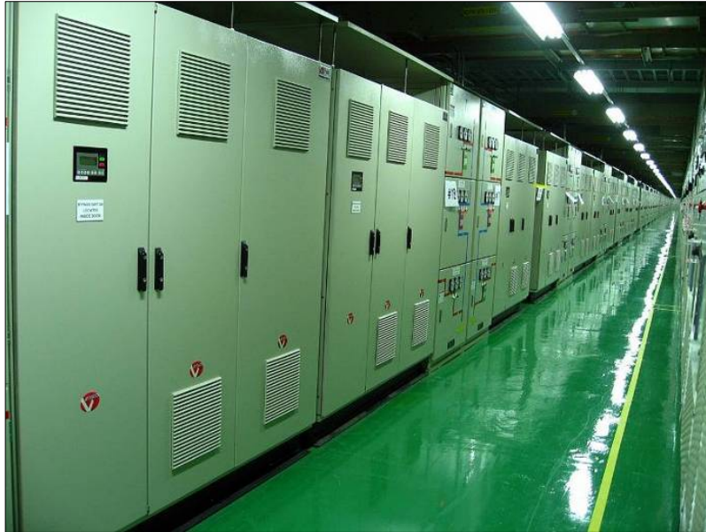
>75MW In Two Plant Rooms Wuxi China
