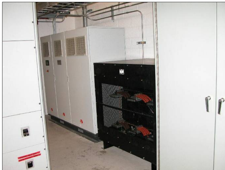
1600kVA AVC installed Aug 2002
