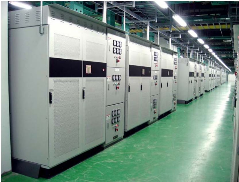
52 x AVC1250kVA Units in Memory FAB, Korea
