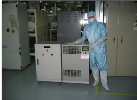
75KVA Protecting Vacuum Pumps
