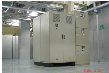
650KVA Protecting semiconductor FAB line
