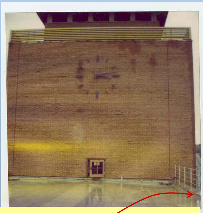
Roof at Bell Labs, Murray Hill, NJ. Card rack was here facing south.
