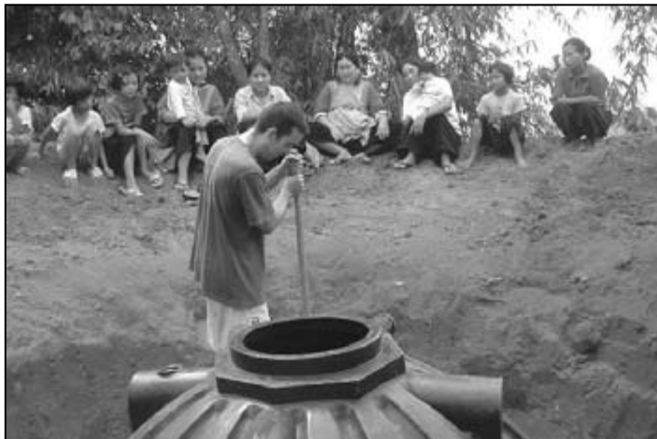
Lisu villagers watch a University of Maryland student work on the installation of a septic system for a new health center.
