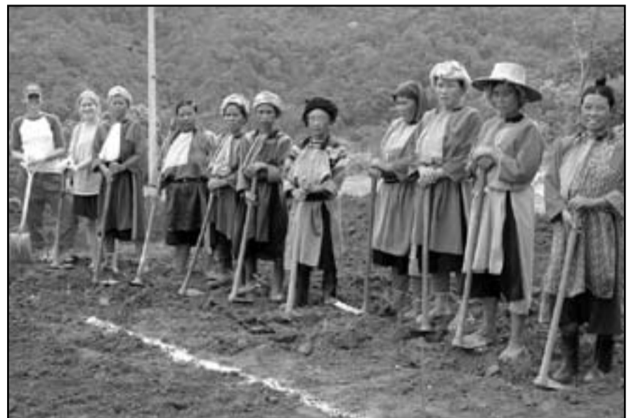
Two student volunteers (left) from the University of Maryland assisted Lisu villagers with the installation of a septic system for a new health center, as part of an Engineers Without Borders project in Thailand this summer.
