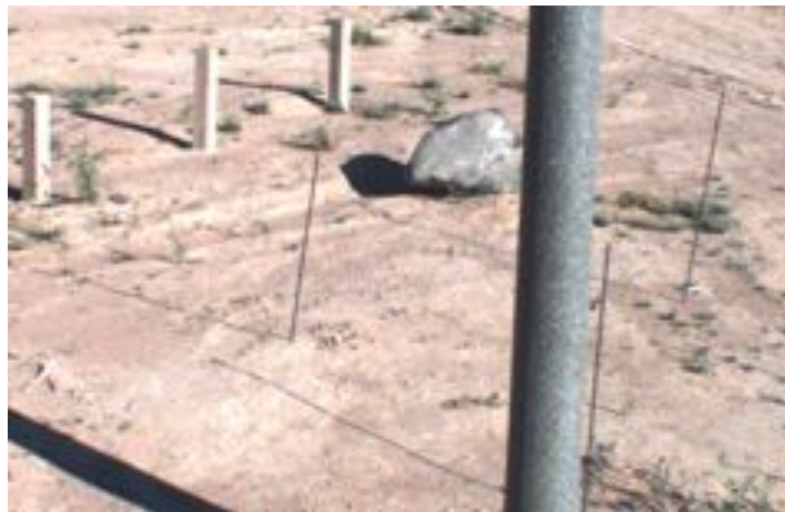
Concrete Telephone Pole
