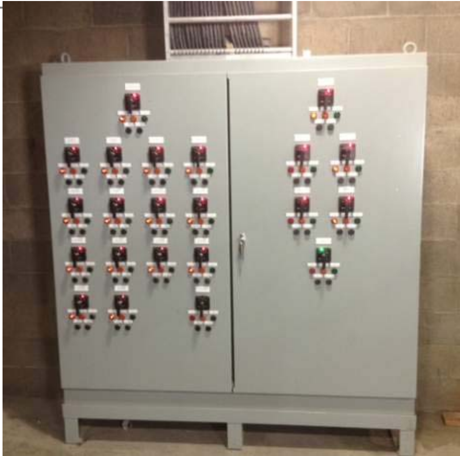
Marshalling panel individual controls for mains, tie and all feeders in a switchgear line-up.
