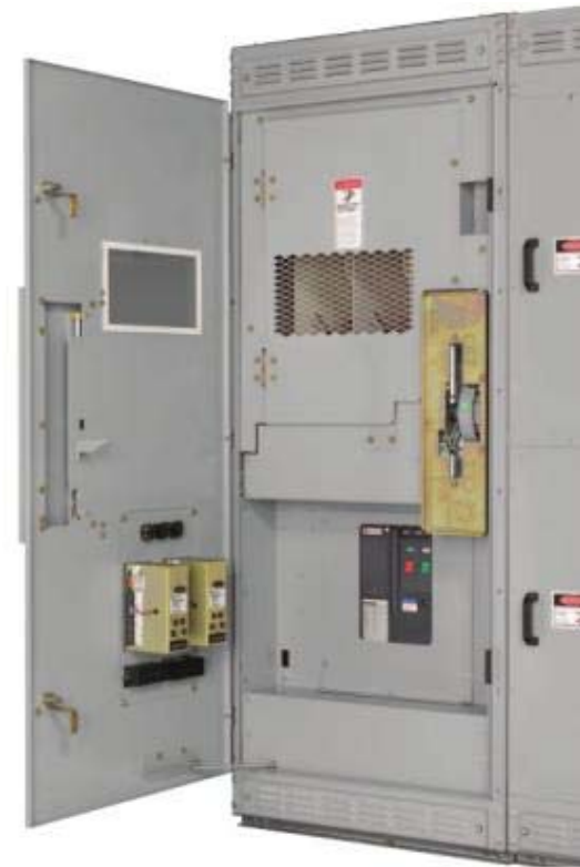
Substation Primary Switch and Vacuum Circuit Breaker
