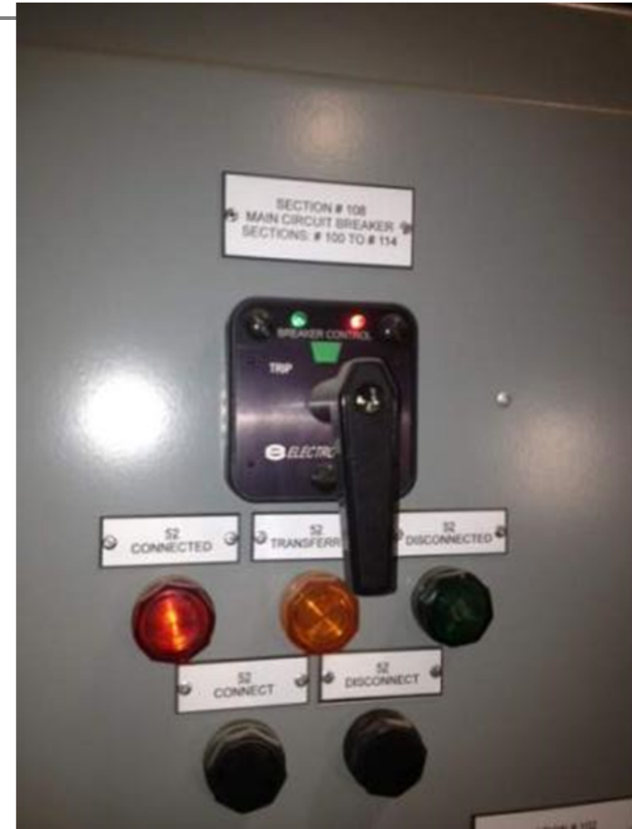
Close-up of individual breaker controls: Open-Close-Trip plus PBs to connect-disconnect and lights indicating Connected-Test-Disconnected
