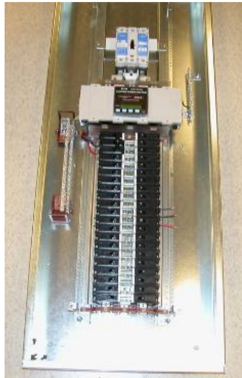
Integrated with Disconnect (~6" of twisted conductor)
