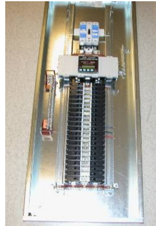
Direct bus connected (No conductor length)
