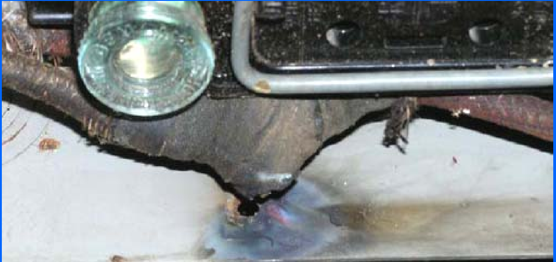
Evidence of Arcing
