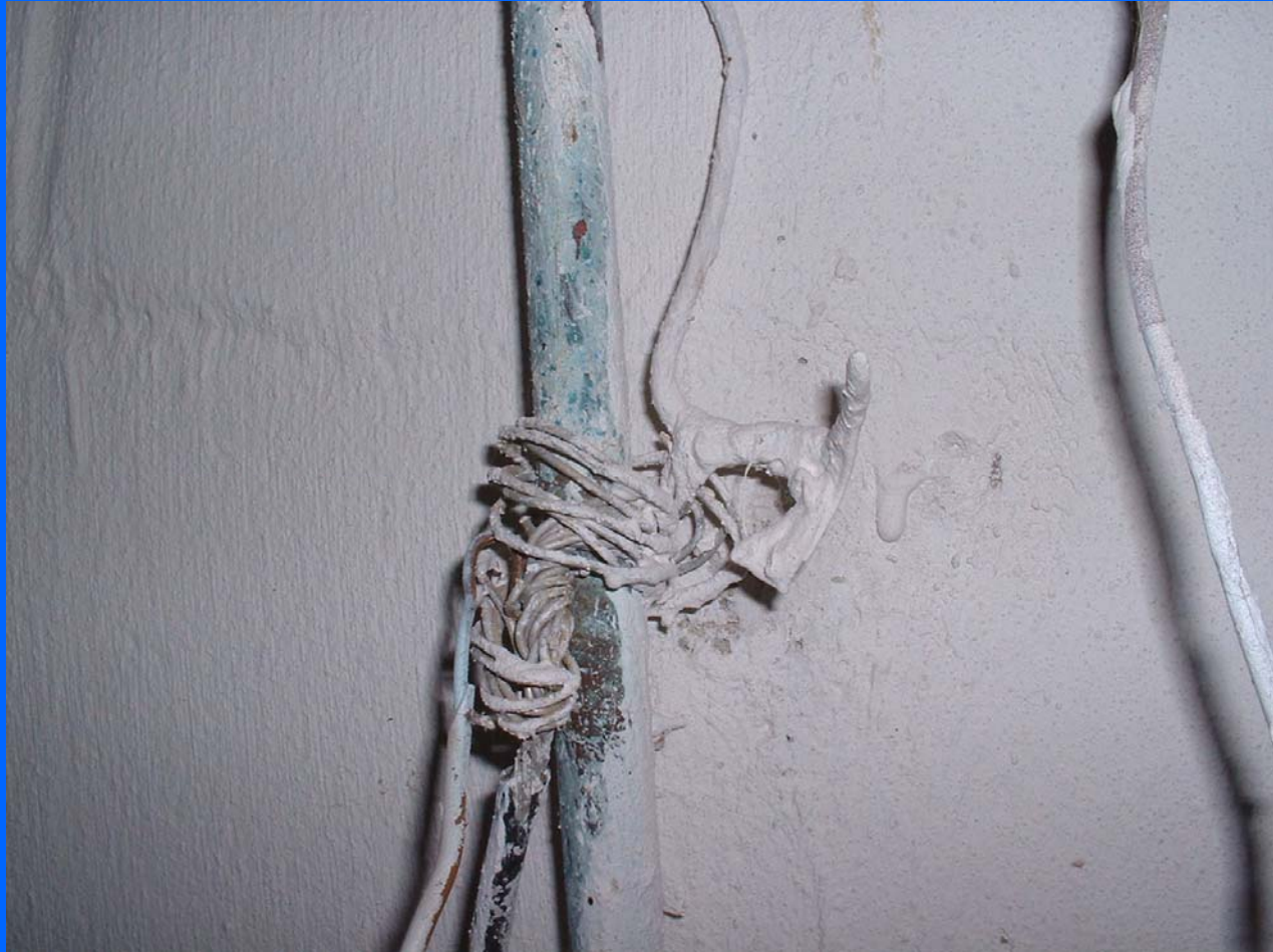
Grounding Electrode Conductor Connection
