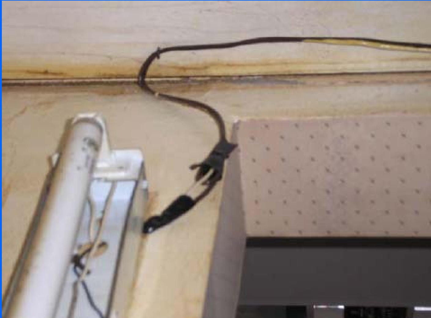
Fluorescent Light Wiring Splice
