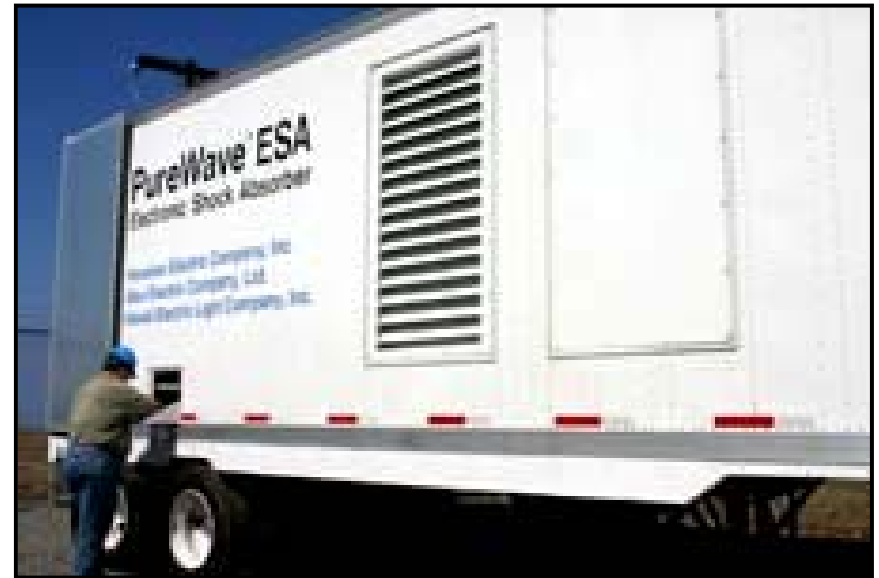
HECO SuperCap Demo (April 2006) Lalamilo Wind Farm Uses Maxwell SuperCaps and an S&C Electric AC-DC-AC Inverter
