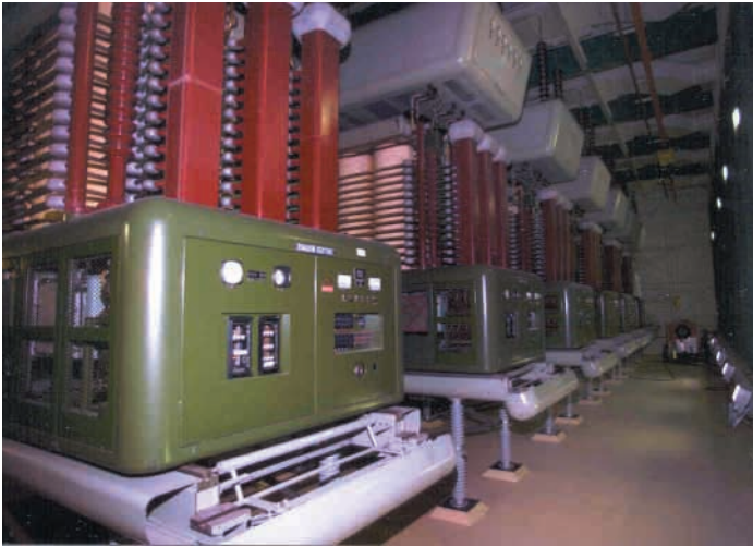
Figure 5: A view of the largest mercury arc rectifier ever built - this type of valve was originally used in the AC-DC conversion stations in the Nelson River DC transmission system. Most of these valves have now been replaced by thyristors. (Source: Manitoba Hydro).
