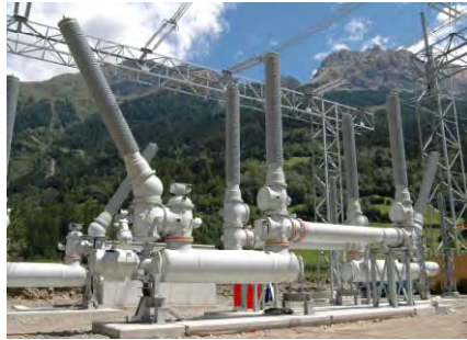
420 kV Substation Robbi, CH: In-Line Configuration
