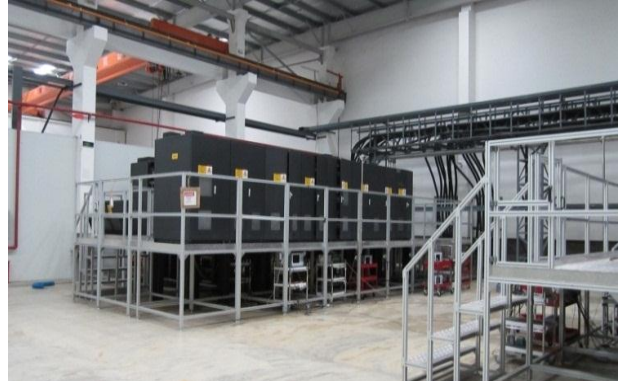
(2) A 30 MVA IGCT converter for Oil & Gas applications
