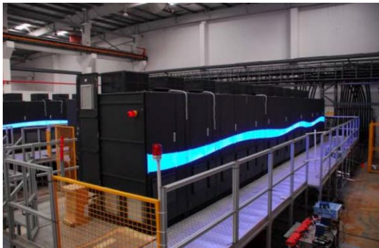
(3) 2x27 MVA machine test bench with four-quadrant pumpback operations
