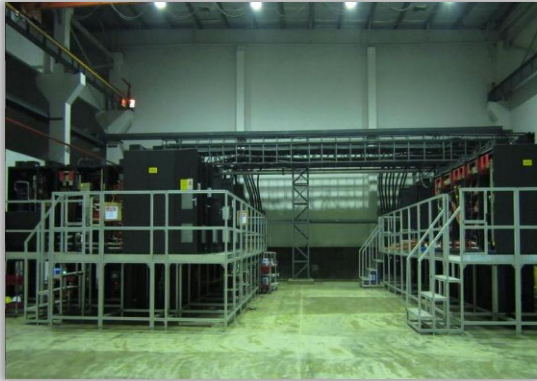
(1) A 11 MW high-speed pumpback VSD tester with 1.25 MW grid
