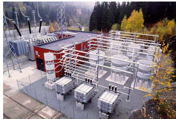
Fig. 11. 420 kV, -160/+160 Mvar SVC in Norway.
