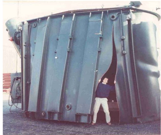
Fig. 1. Transformer tank rupture (extracted from [1])
