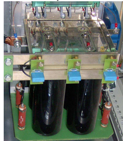
Fig. 10. DC bank of the voltage source converter
