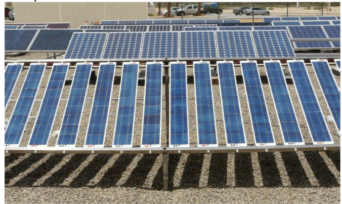
Fig. 2. PV panels under test in Abu Dhabi.
