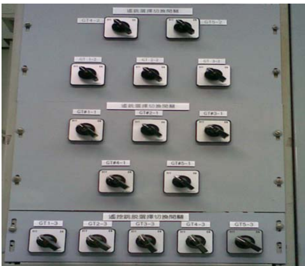
Fig. 5. Generators tripping control panel of the first stage SPS
