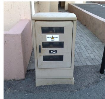
Fig.1 Customers distribution box
