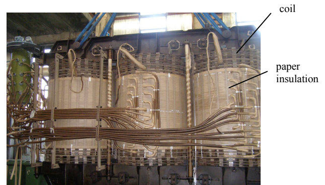
Fig. 4. Coils of transformer
