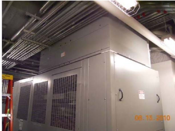
12.47kV snubber mounted horizontally above transformer
