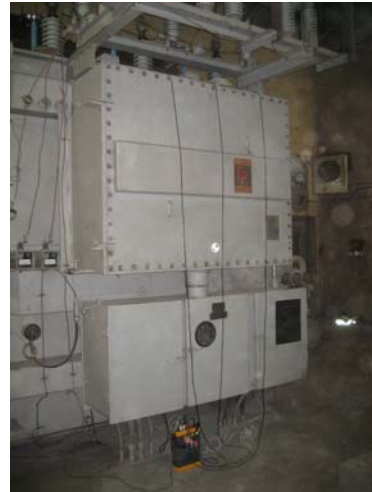
PQ Meter and Test Leads
