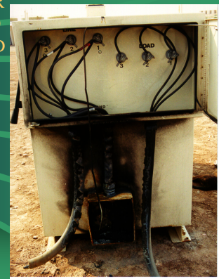
MOTOR STARTER FAILURE DUE TO ARCING GROUND FAULT
