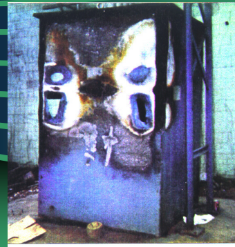
SWGR TAP BOX FAILURE DUE TO ARCING GROUND FAULT
