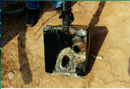
TVSS Failure Due to Arcing Ground Fault
