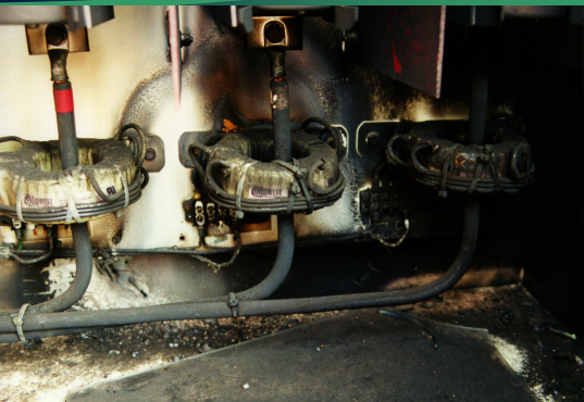
MOTOR STARTER FAILURE DUE TO ARCING GROUND FAULT
