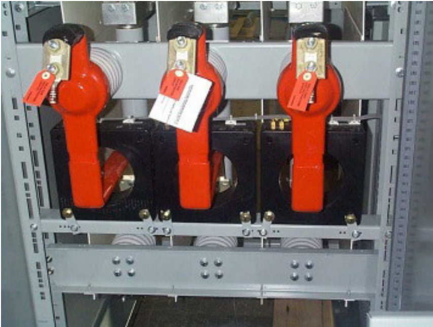
Normal metal-clad cable terminations
