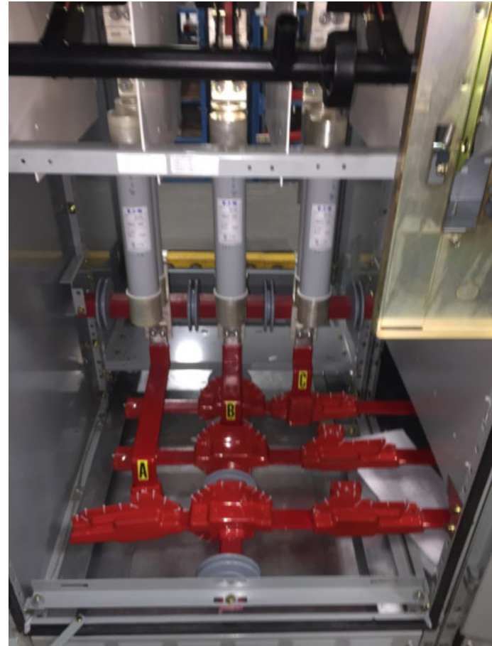
Metal-enclosed switchgear with insulated bus option
