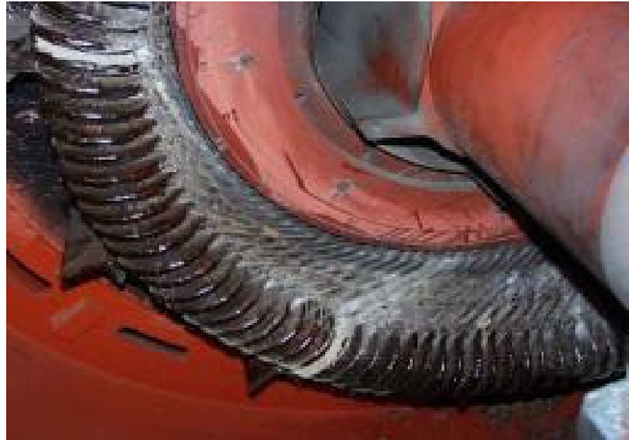
Partial discharges on motor stator
