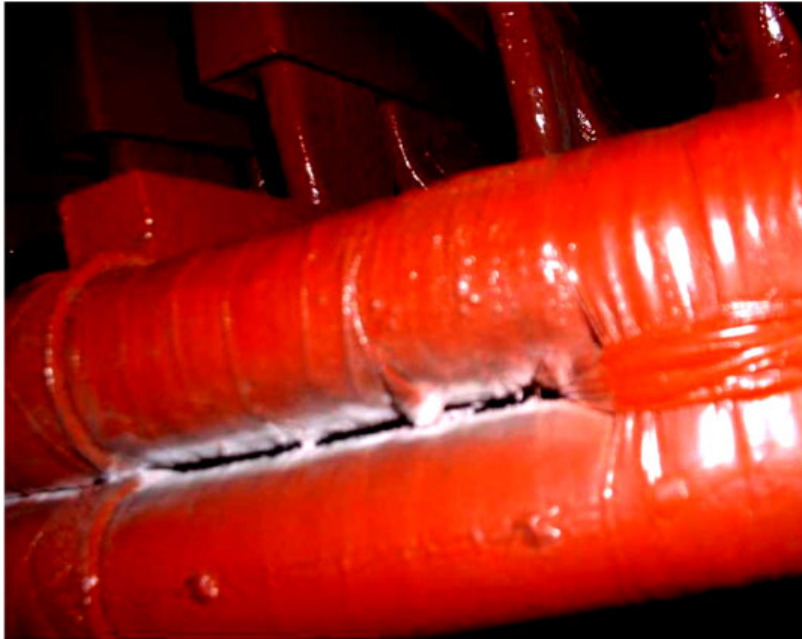
Phase to phase discharges on ring bus
