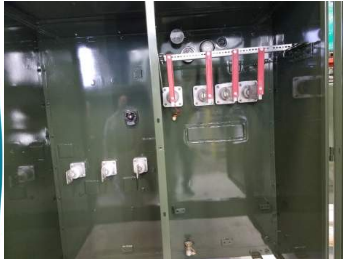
15kV / 480V Transformer compartments
