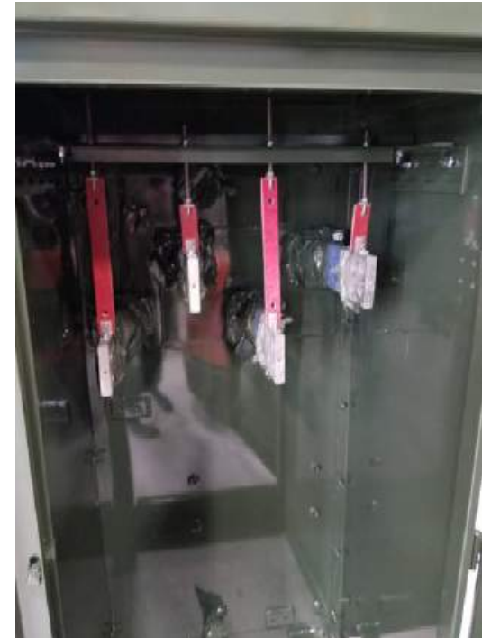
480V Transformer compartments
