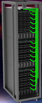
(RACK OF SERVERS)
