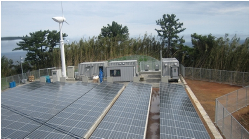
Kyushu Japanese Microgrid System
