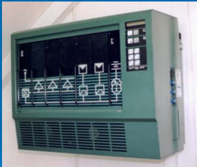
Practical realisation of a Central Control Station for an autonomous Photovoltaic System.
