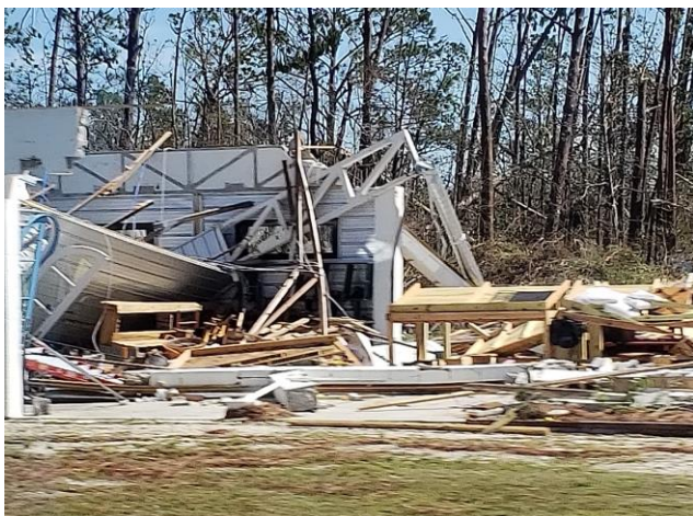
Damage from hurricane Michael
