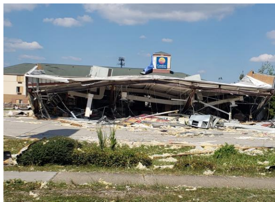
Hurricane damage after hurricane Michael
