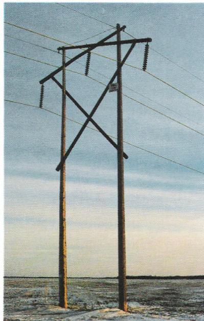
Figure 1: 230 kV Gulfport woodpole transmission line structure.
