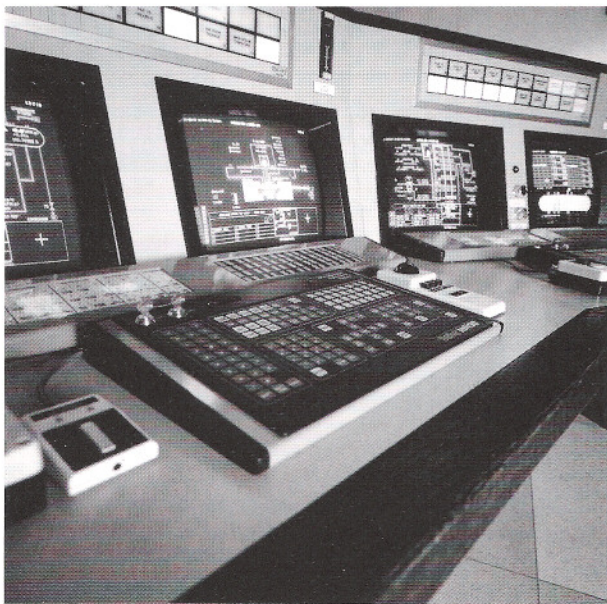
Figure 2. Shand has two control rooms: one to monitor the water treatment system and the other, made up of six work stations (above), controls the remainder of the station's operations.
