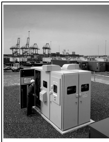
Figure 4: This partnered AVC installation is saving the Seagirt Marine Terminal in Baltimore roughly $220,000 US annually in demand and PF charges, and at the same time freeing distribution capacity for its utility Baltimore Gas & Electric. (Seen in the photo is Ed Wilson, Project Engineer with Constellation Energy Source, a premium power group of BGE).
