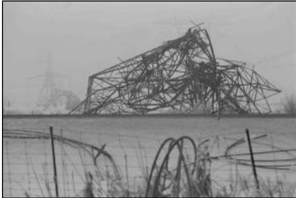
Figure 1: Damage to overhead line by ice accumulation in 1998
