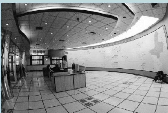
Figure 1: Ningxia Autonomous Region Generation Control Centre, China.
