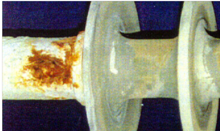
fig 1 Example of deterioration affecting the metal end-fitting: Flange Corrosion [11].
