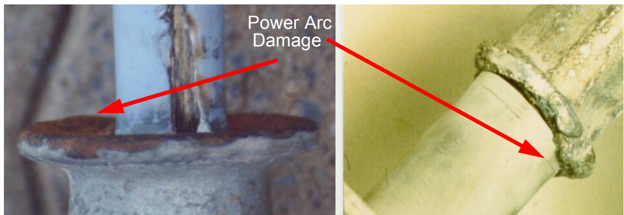
fig 2 Examples of damage occurring on the metal fitting: Power Arc Damage . Right photo [11].
