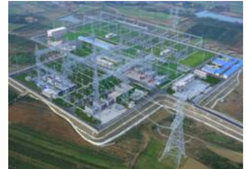
China 1100kV projects
